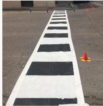
A connectivity demonstration is installed in a downtown area
