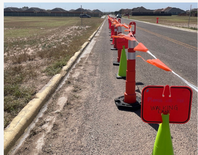
Protected walking lane installed while pilot-testing connectivity components from a middle school to the adjacent park and neighborhood
